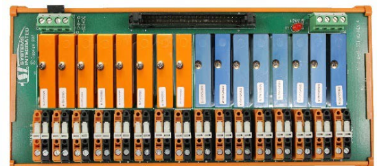
FIELD TERMINATION INTERFACE BOARD WITH MODULES
